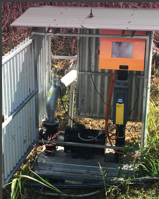
Photo: The Davey well pump – 7.5kW ISO CM 80x65-160 with a variable speed drive (VSD) was the ideal efficiency match for Rex's lateral irrigator.
